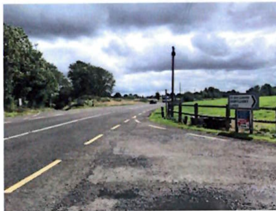
Photo 01: View to the south with ESB pole, concrete post and rail impeding the sight line.
